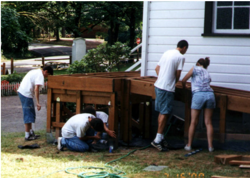
Troop 611 scouts — led by Scout Jim Guntermann — added a wheelchair ramp to the historic pioneer church to bring modern accessibility to the classic structure.
